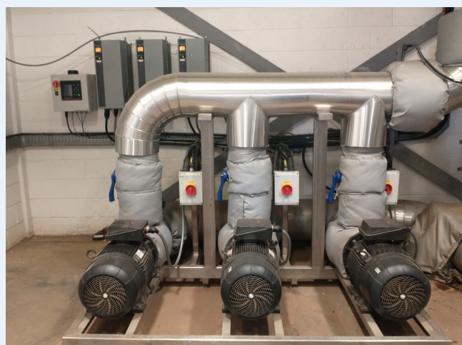
Figure 7: The Grundfos team advised Arla Foods on the selection of smart pumps and controls, and delivered a turnkey end-to-end system for cooling and ice water. This included the installation, pipework and commissioning, and validation of the savings.
