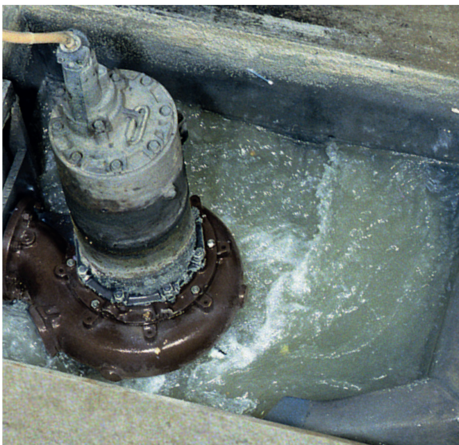
Sewage pump with immersible motor in wet well
